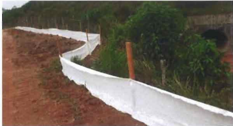
Silt fences are installed prior to the commencement of work on a site
