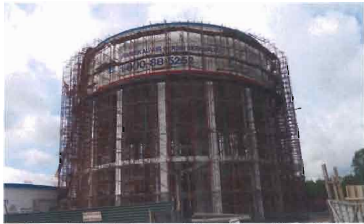
An elevated water tank constructed by our Group at Bandar Sultan Suleiman, Selangor
