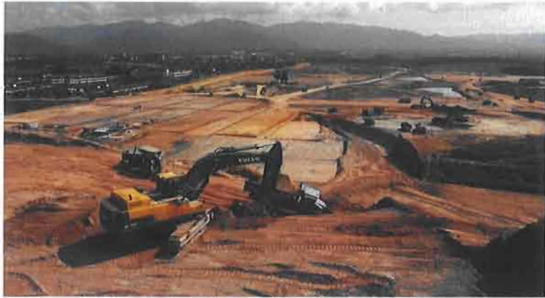
An excavator, dump truck and back pusher are involved in the excavation and fill process
