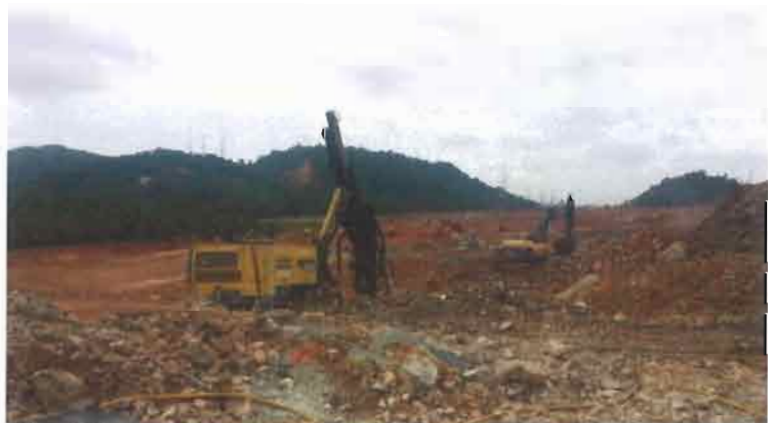
Step 2: Drilling works undertaken by inserting ammonium nitrate and explosive material deep into the ground
